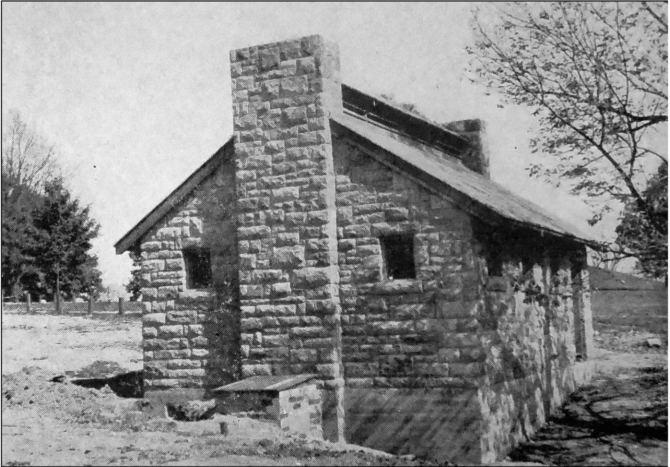
Figure 8. Restroom being constructed at Serpent Mound, c. 1934, by the Federal Emergency Relief Administration Transient Division (Photo Credit: Dick Dreyer in State Relief Commission of Ohio and its Activities , 1935)
